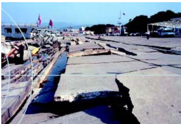
Figure 11: Damage to the main pier and seawall at the Golcuk Naval Base
